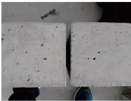
图13 出入泵硬化混凝土气泡 (图中左右试件分别为入泵和出泵取样) Fig.13 air bubbles on surface of hardened concrete before and after pumping
